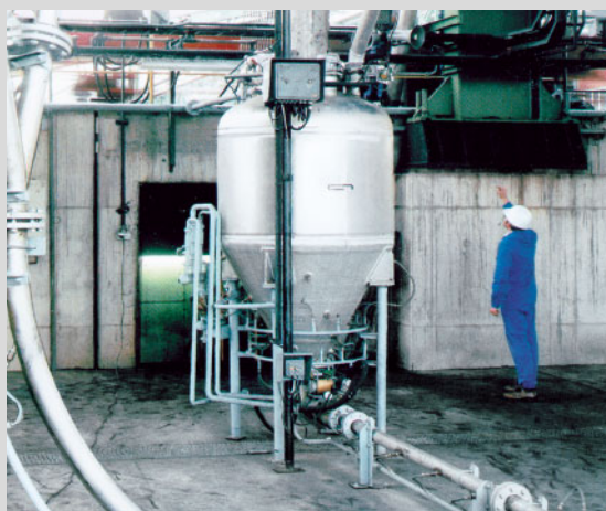
1) Pneumatic conveyor system for carbon blacks
