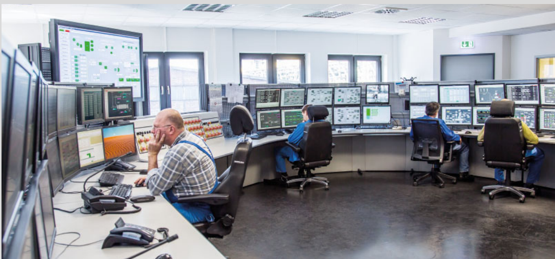
Figure 29: Control room of a carbon black plant
