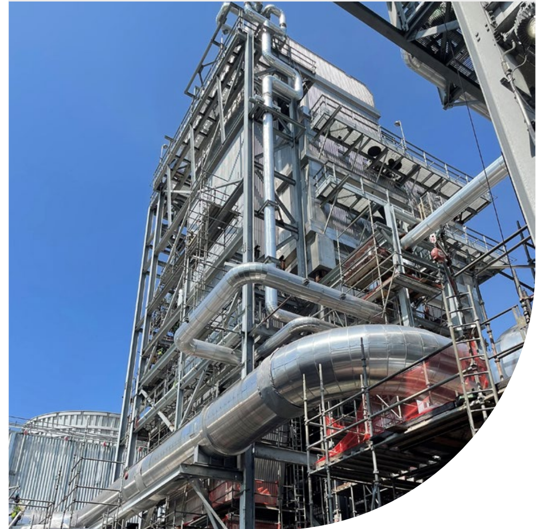
Orion's plant in Ivanhoe, Louisiana.
